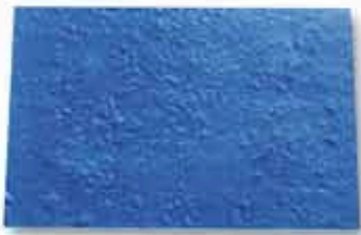
Piedra erosionada/ 585 x 390 mm
